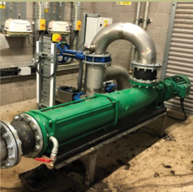
BIOMASS RECIRCULATION PUMP
