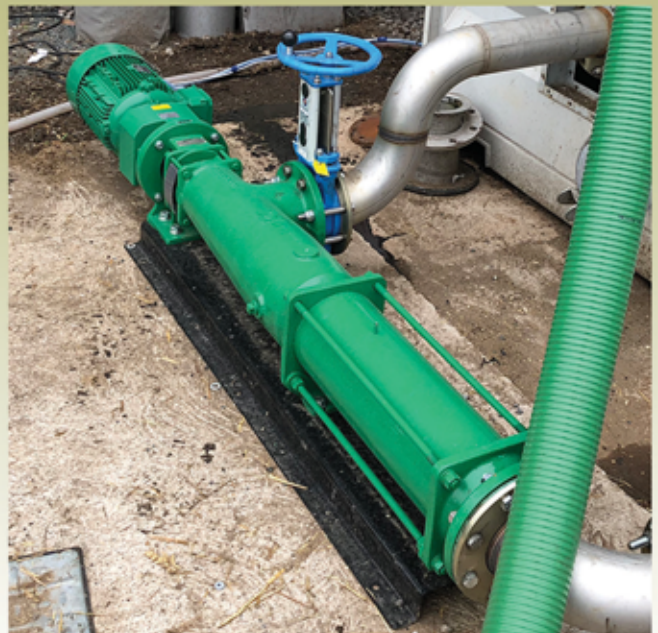
BIOMASS TRANSFER PUMP
