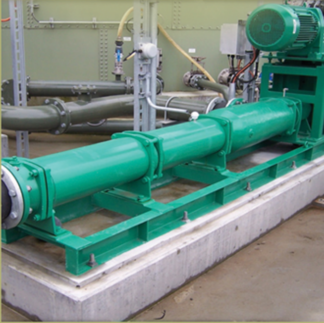
DIGESTATE TRANSFER PUMP
